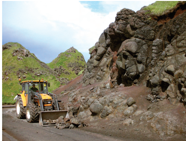
National Trust clearing debris from a recent slope failure (photo provided by National Trust)
