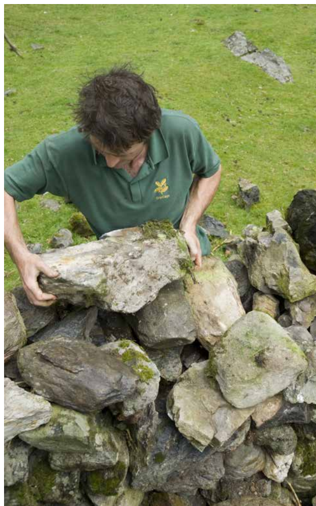
Repairing the traditional dry stone walls at Hafod Y Llan farm, Snowdonia © NT Images/Paul Harris
